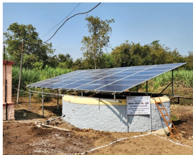
Harnessing solar energy
